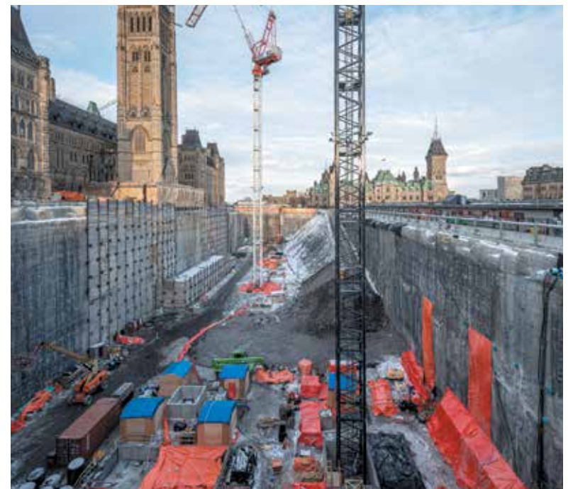
The Parliament Welcome Centre pit where two of three planned tower cranes have been installed as of January. Photograph courtesy of Public Services and Procurement Canada
