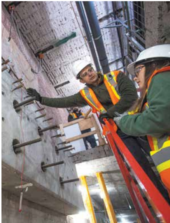
PSPC's Siavash Mohajer points out a concrete sandwich beam that will be part of the support network holding up Centre Block during an exclusive Hill Times tour of the site this past February. The Hill Times photograph by Andrew Meade
