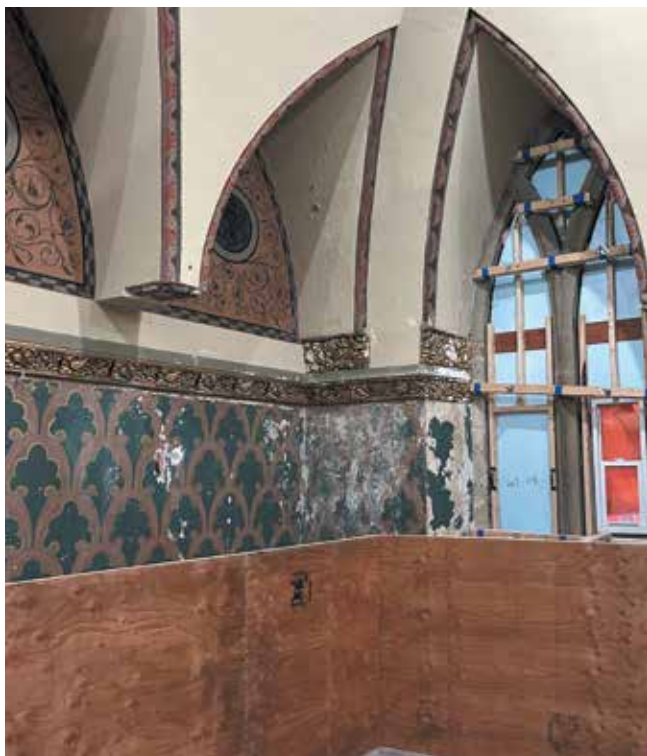
An area with particularly bad water damage in the House Speaker's dining room. The Hill Times photograph by Laura Ryckewaert
