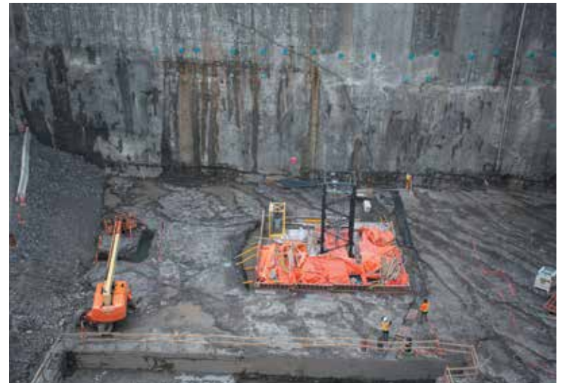
The base of one of three tower cranes that will be installed for construction of the underground Parliament Welcome Centre. The Hill Times photograph by Andrew Meade
