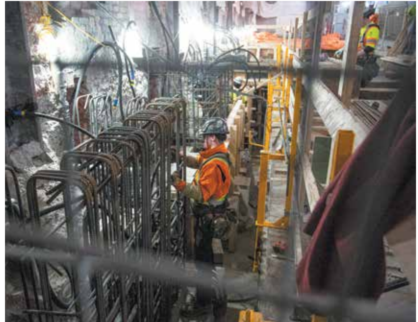
Level 1 slab replacement work in progress on the west side of Centre Block on Feb. 7. The Hill Times photograph by Andrew Meade
