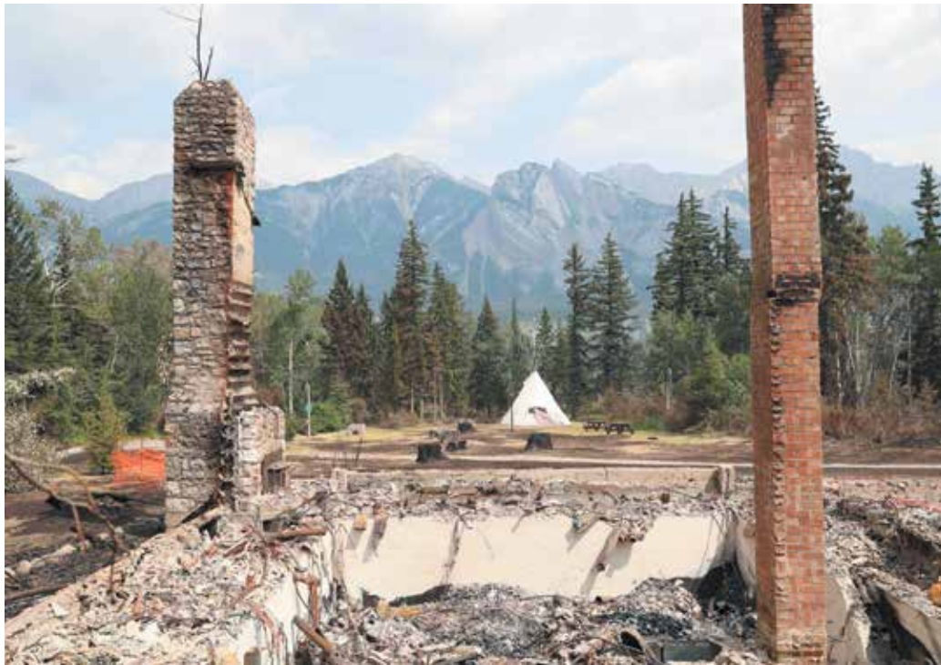
The remains of the Palisades Centre in Jasper National Park after a July wildfire. The inaugural Canadian Emergency Preparedness and Climate Adaptation conference discussed the future of this country's disaster resilience. Photograph courtesy of Parks Canada
